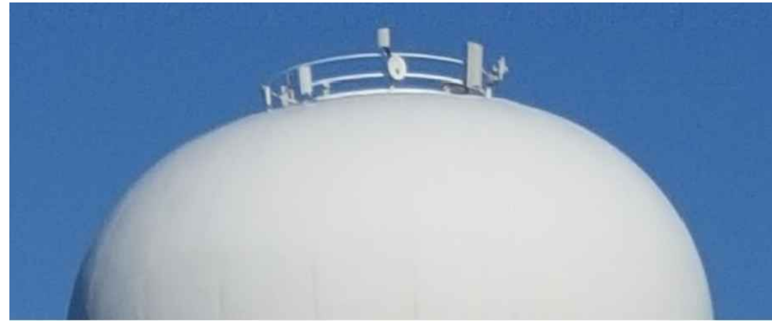
EXISTING INVISALINK EQUIPMENT ON TOP OF TOWER AND INSIDE BELL TO BE PROTECTED DURING CONSTRUCTION. CONTRACTOR TO COORDINATE WITH CITY OF OWOSSO AND INVISALINK.
